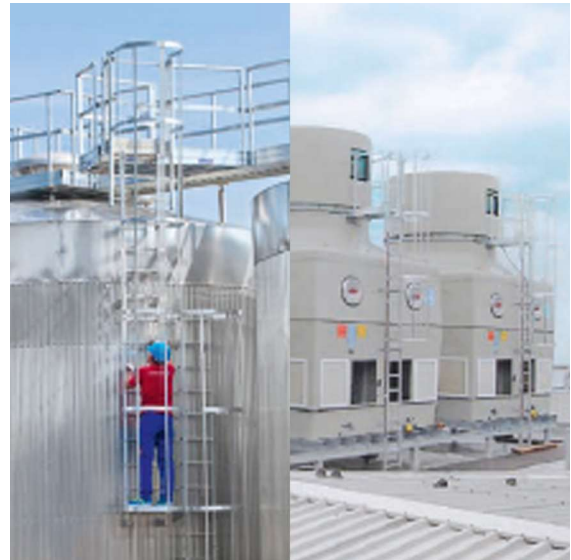
Ladder for plant machinery maintenance, Hymer 3385 EN ISO 14122-4
